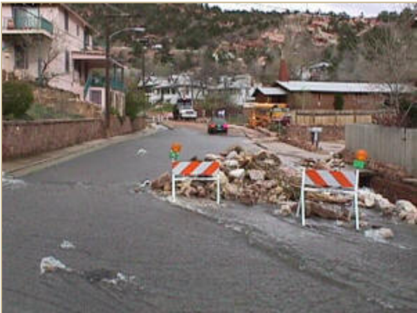
Canyon Avenue in Manitou Springs
