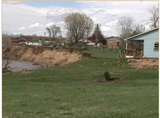
Erosion caused by Fountain Creek (the yard used to go to the left edge of the photo)
